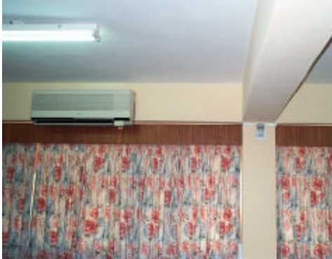
Passive Infra-Red Sensors to control lights and AC
