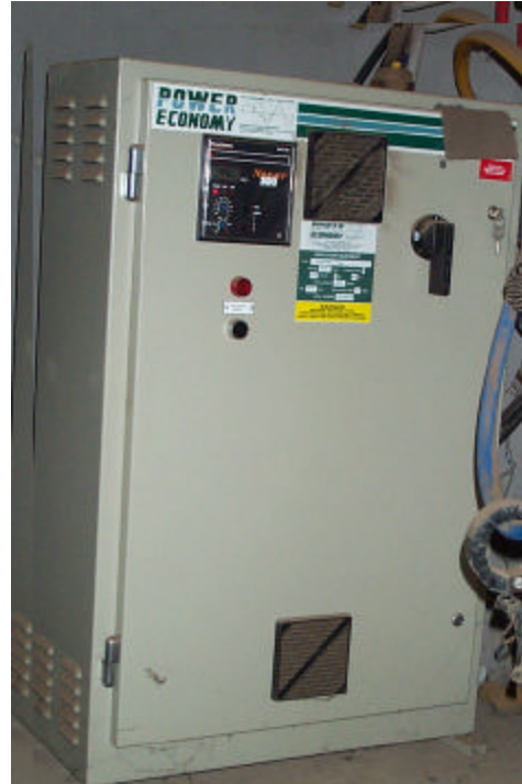
Capacitor Bank, installed at MOME
